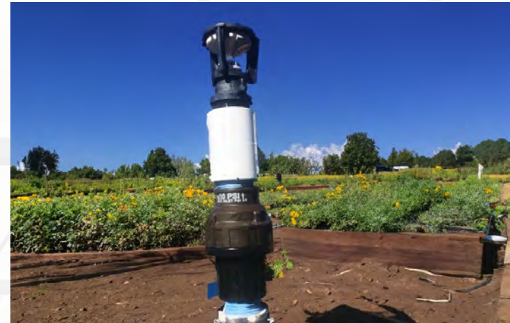
Fig. 1. This sprinkler was equipped with a 20 psi pressure regulator.
